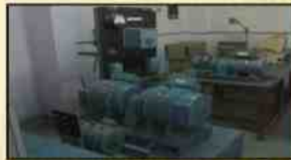
CONTROL SYSTEM LAB
